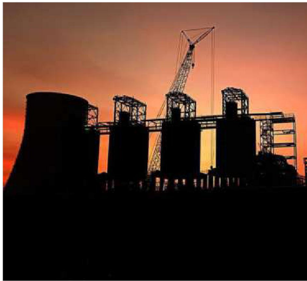
READY TO GO. Gas-based plants will first offer their power to the power purchase agreement holders SIVA SARAVANAN S
